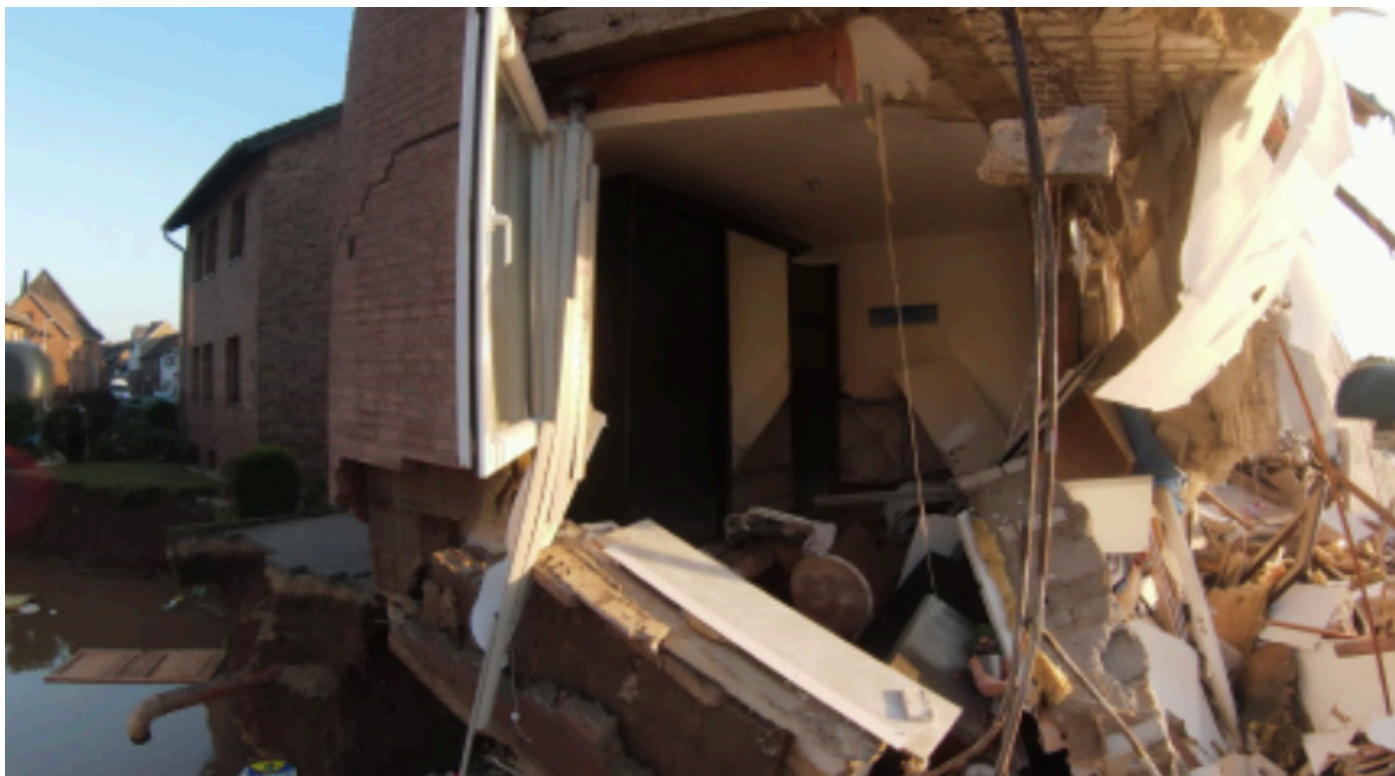
Figure 21: Flood damage to building - Deployment of aerial robots during the flood disaster in Erfstadt / Blessem, Germany (Figure 8 in Surmann et al. 2022).
